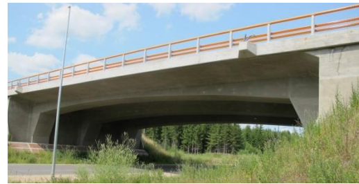
Fig. 9. Cross section and elevation of bridge on road E22 over road V920. FE model
