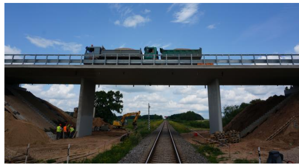
found when vehicle crossed bridge
